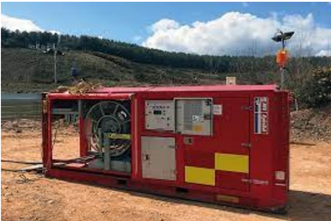
Figure 4 - High volume pump
